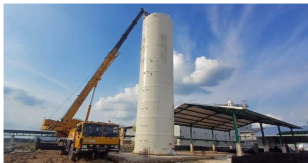
Figure 8. The field erection and integration phase of the FRP Scrubber tower and its anchoring system.
